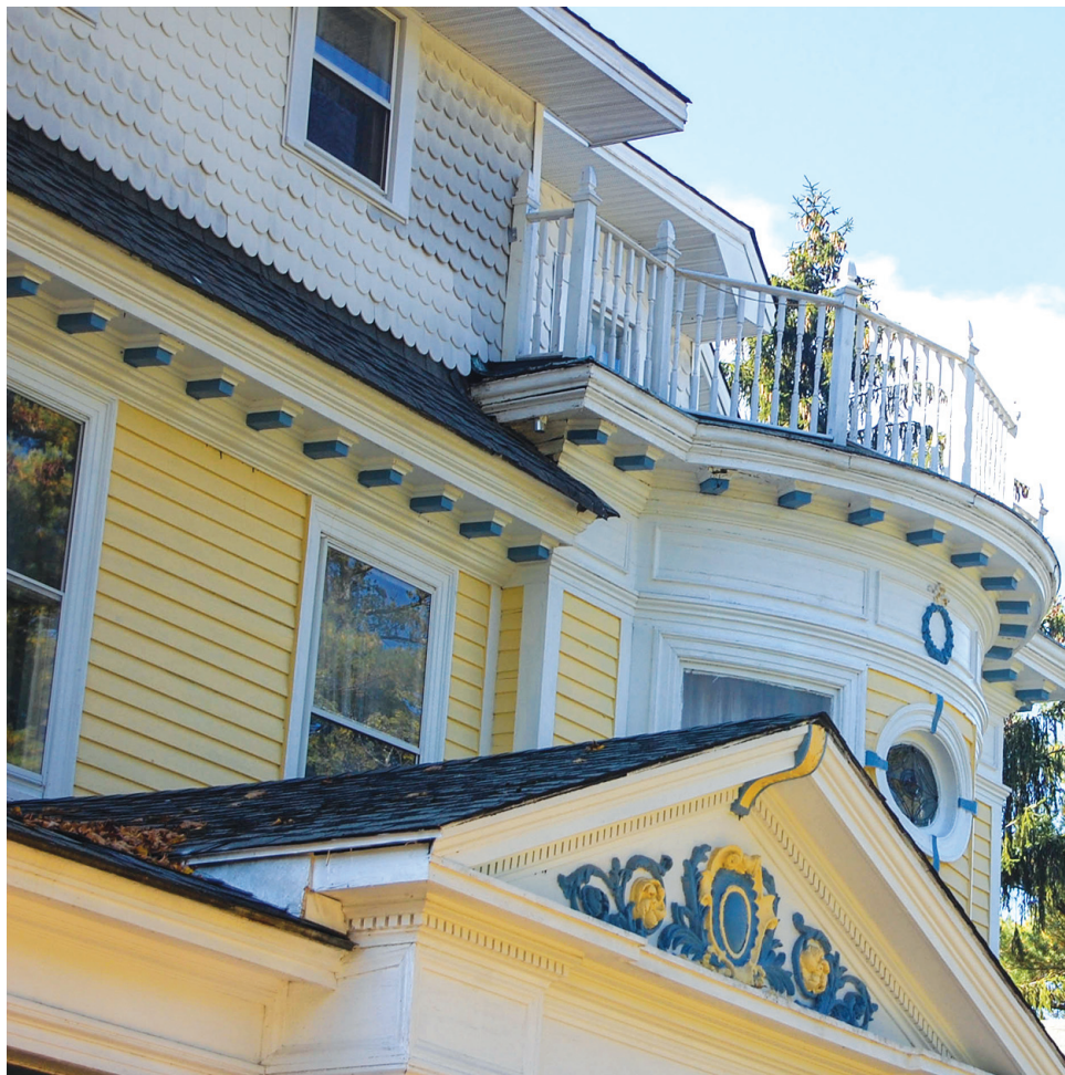
Victorian details have been brought back to their original splendor at of Burn Brea Mansion in Glen Spey, NY.
